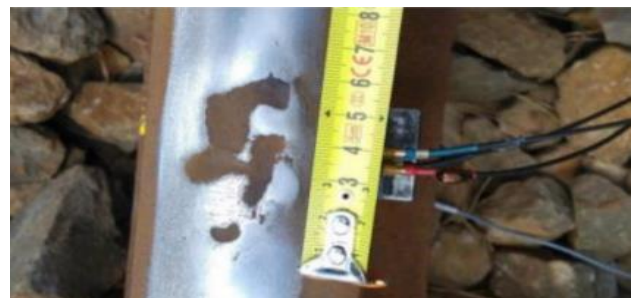
Fig. 3. Example of a "squat" defect [8]
